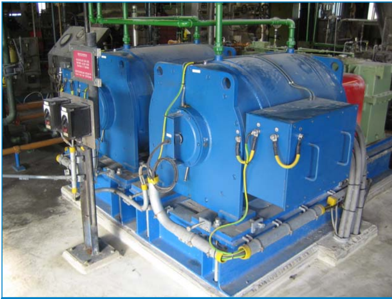
Subject : 750 kW - 640 rpm - 520V - IC 41W Application : Mixer drive Installed : 2006
